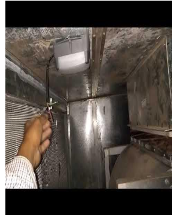
Limit Switch for AHU Room & Fire Shaft Door
